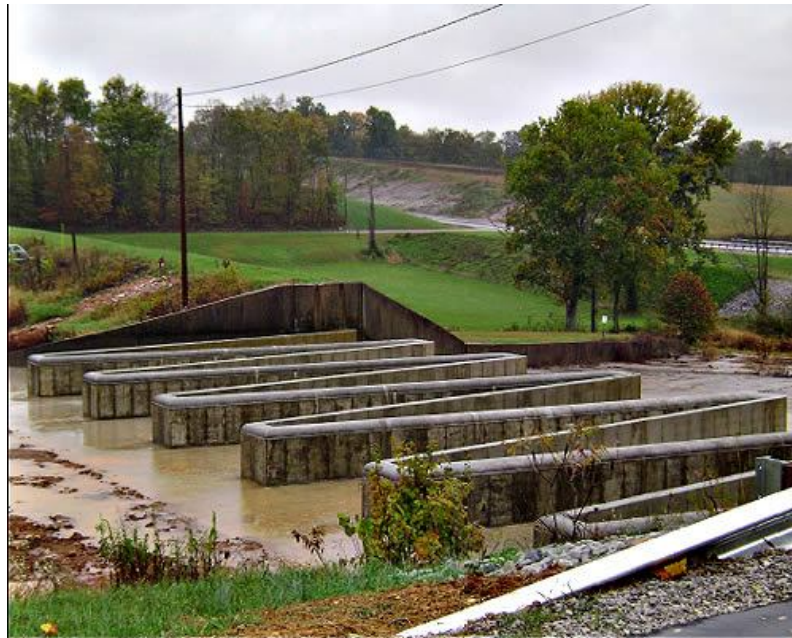
Figure 6 - Typical Labyrinth Spillway (Lake Salinda Dam Improvements, n.d.)
